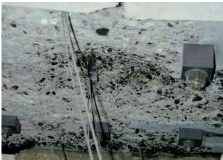
Figure 6.5: Spalling-off of the concrete cover /1/
